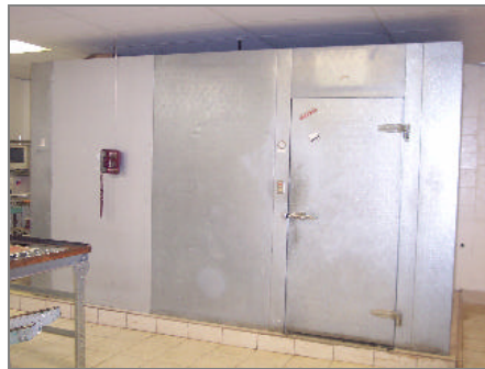
Figure 1: Prepreg storage room
